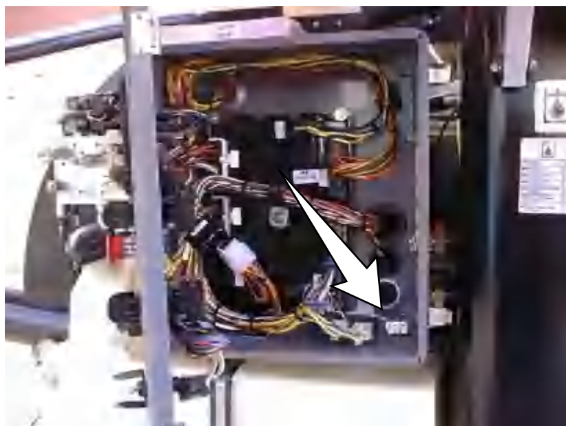
GROUND CONTROL CONNECTION
